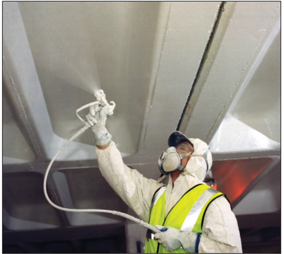
Concrete repair and protection work should always be entrusted to specialist contractors such as CRA members. (Pic by kind permission of Concrete Repairs Limited)
