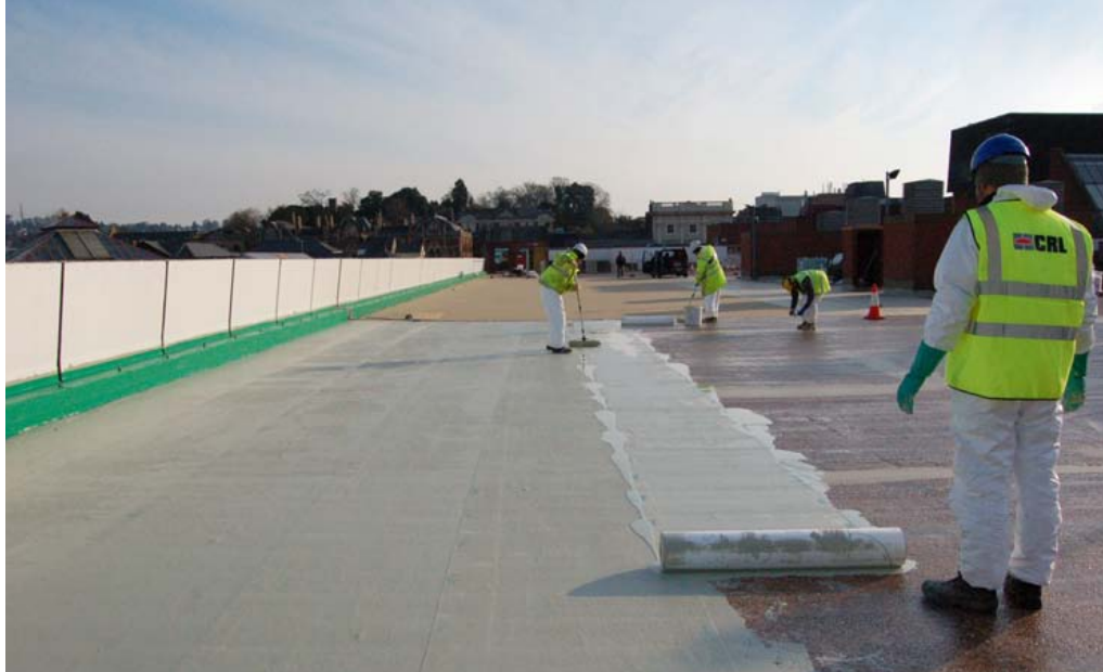
waterproofing the top deck of Guildhall Multi-Storey Car Park, part of the Harlequins Shopping Centre in Exeter
